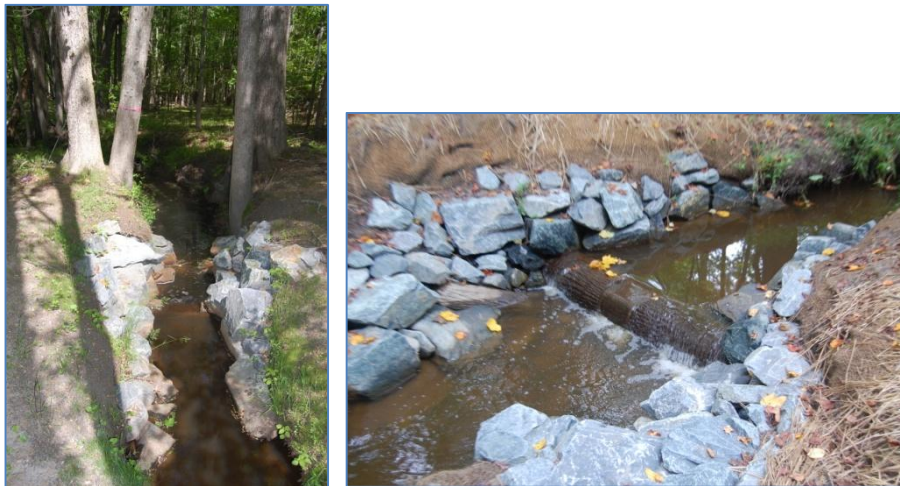
Figure 13: "Log vane 3" converted to log drop (April 2010 on left and August 2009 on right)
