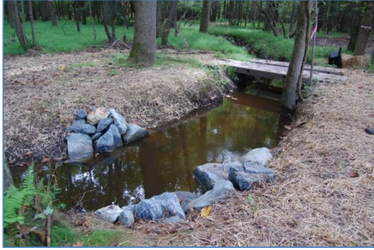
Figure 14: Log vane #7 is buried due to back water from downstream log drops. (August 2010)
